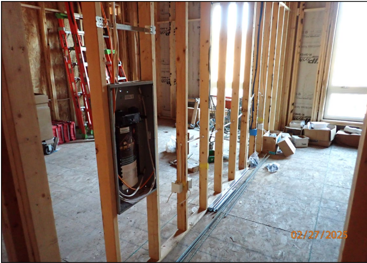
22 3rd Fl., Electrical panel
