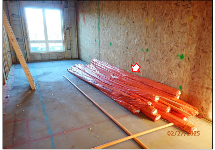
Fire sprinkler pipe materials on site
