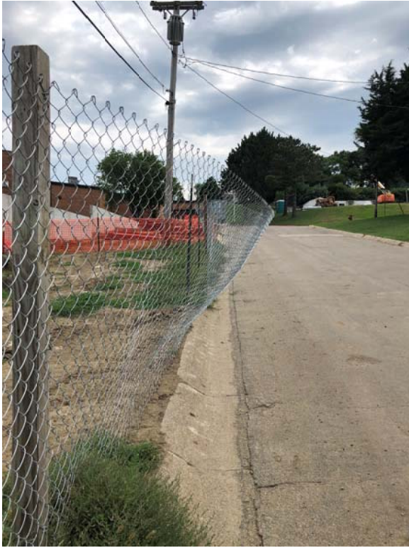
Reattach fence to posts
