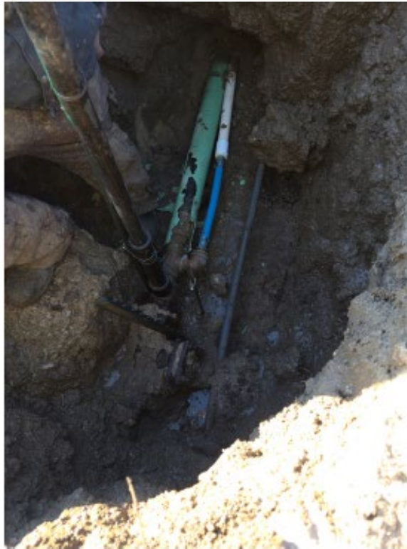
EXISTING YARD HYDRANT PIPING AT VALVE
