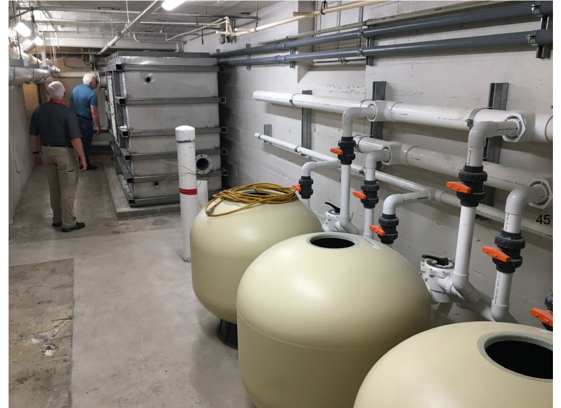
New sand filters and surge tank
