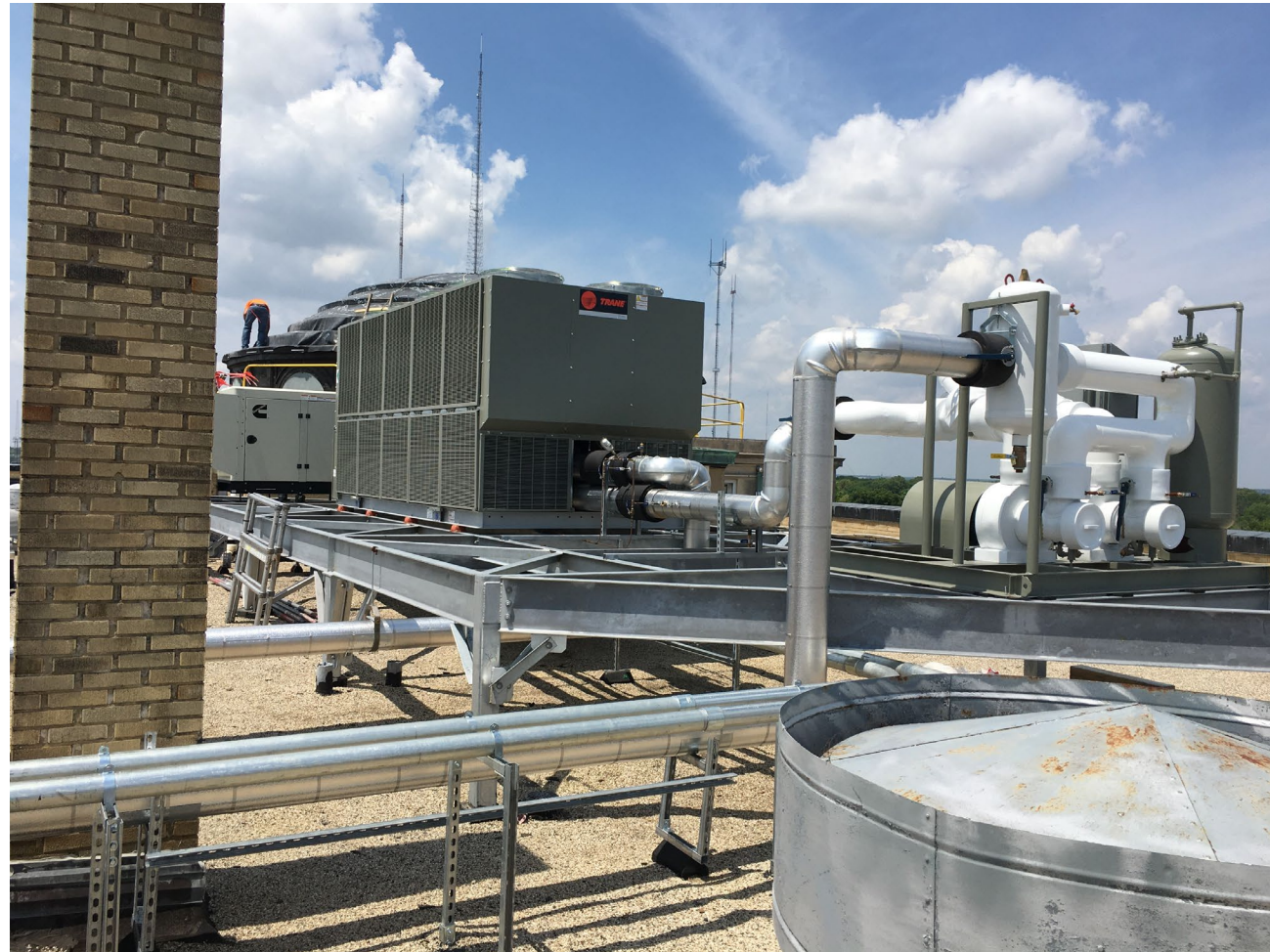
New chiller is now in use
