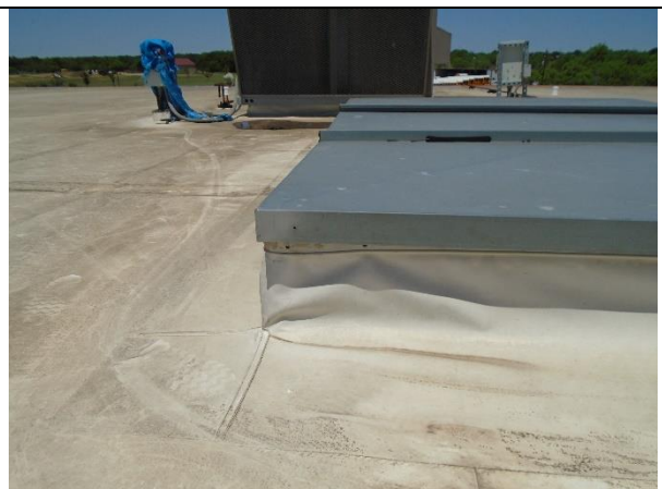
Curb flashing is failing and the cap is not properly secured.
