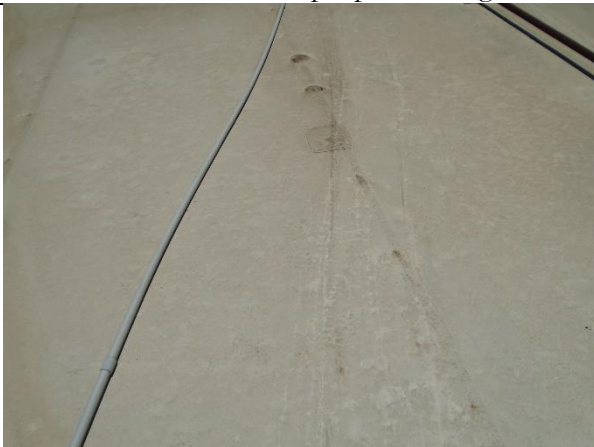
Loose condensate is damaging the membrane and will lead to leaks.
