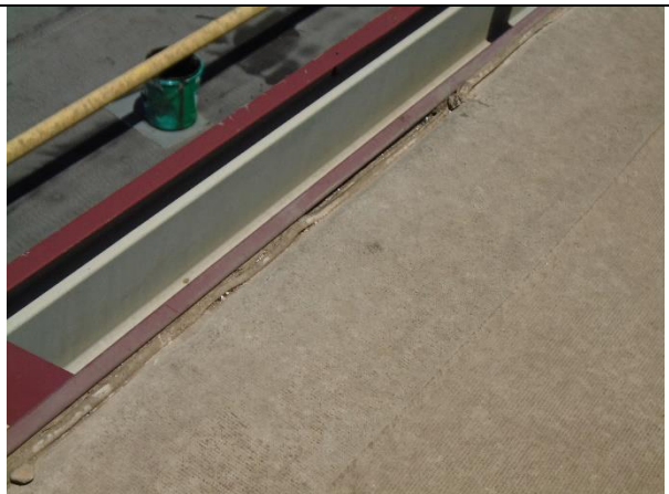
Membrane is pulling the gutter metal causing separation and leaks.
