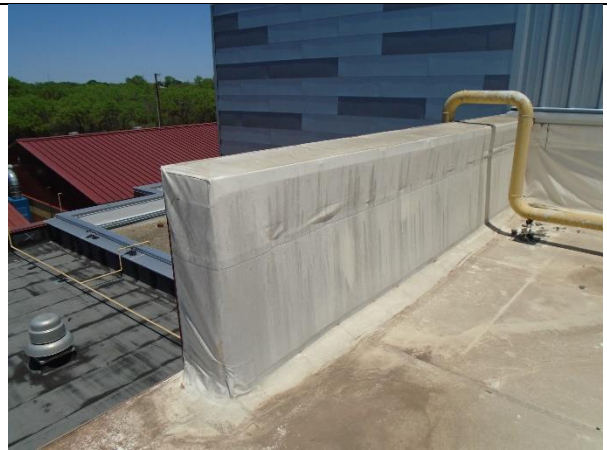
Wall flashing is failing. (Typical)
