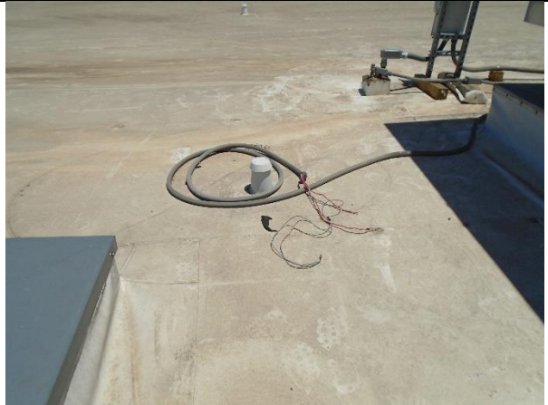
Abandoned penetrations should be eliminated to reduce the chances of leaks.
