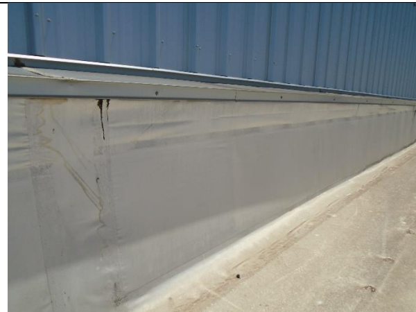
Wall flashing is failing and is starting to pull at the metal in several areas.
