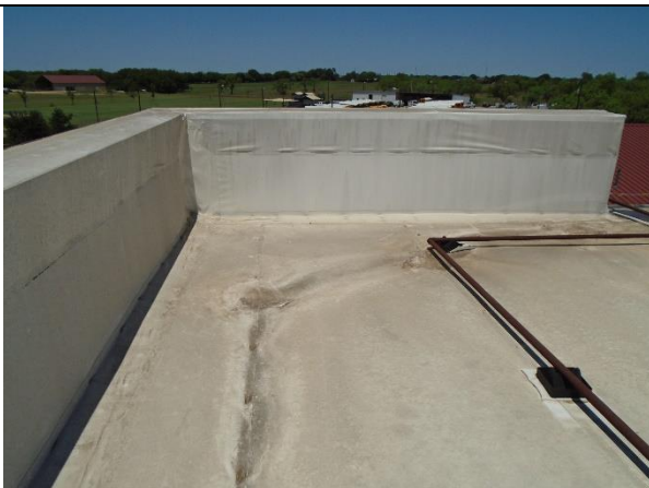
Failing wall flashing. New taper will be installed in the corners for proper drainage.
