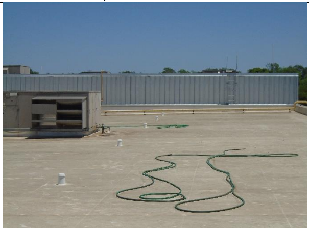
Loose debris and or equipment will lead to membrane damage.
