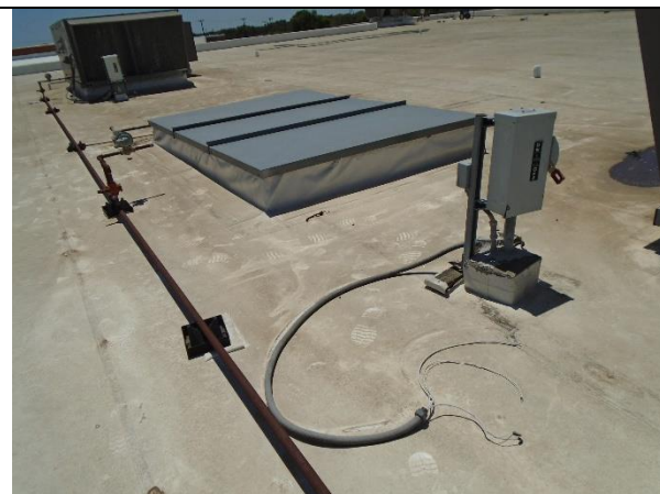
Abandoned penetrations should be eliminated to reduce the areas for water infiltration.
