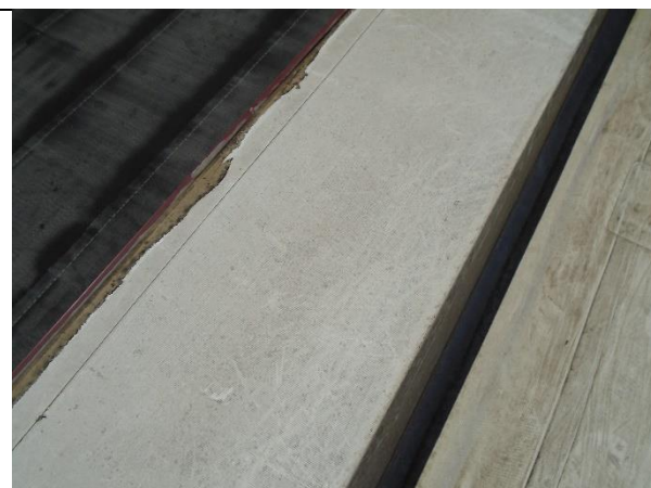
The membrane was installed over the metal coping. Existing repairs were noted.
