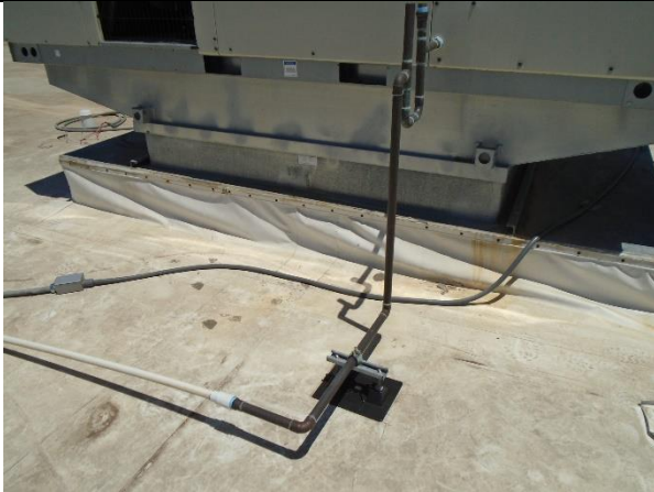
Curb flashing is failing. (Typical)
