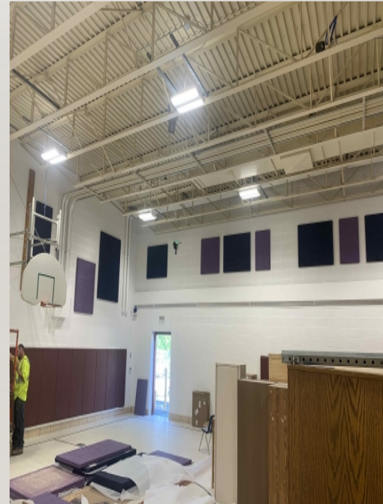
ECFC Area B Gym Paint / Acoustic Panels
