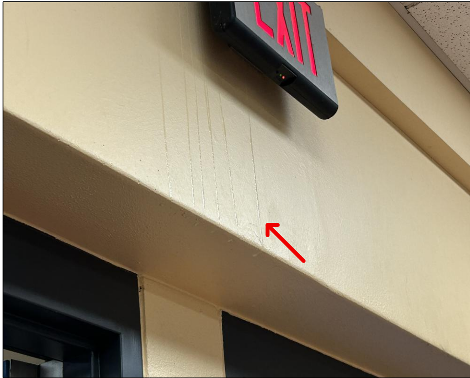
Water intrusion at failing vertical control joint at the time of the water test.
