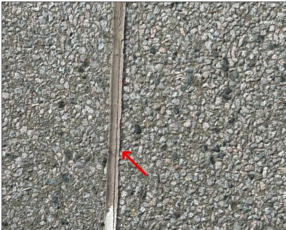
Failing sealant at vertical control joint.
