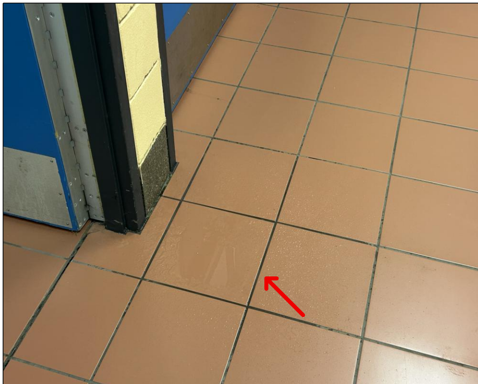
Water intrusion at vertical control joint at the time of the water test.
