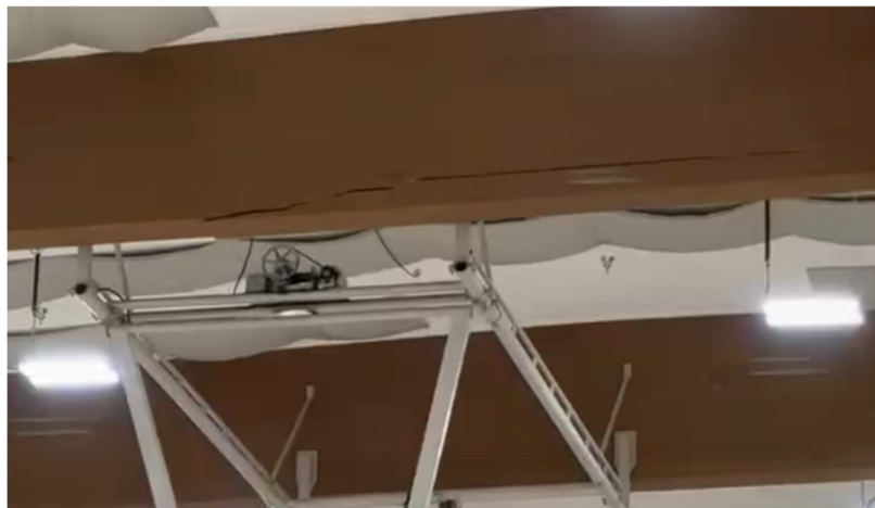
Figure 1 – Beam A Initial Failure
