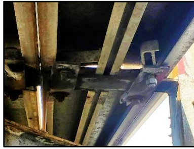
Loose/misaligned clip sets.
