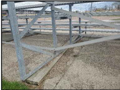
Misaligned/bent frame member.
