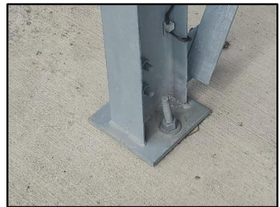
Concrete ground anchor.
