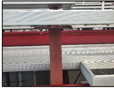
Damaged seat support.
