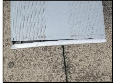
Loose/damaged end cap.
