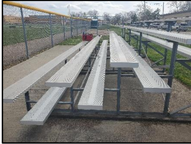
Missing side/rear guardrail fencing.
