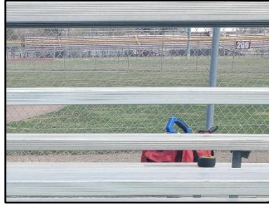
Gaps between planks exceed 4" standard.
