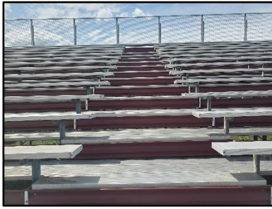
Missing mid aisle handrails.
