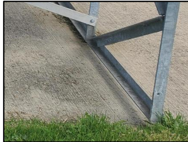
Missing ground sill.
