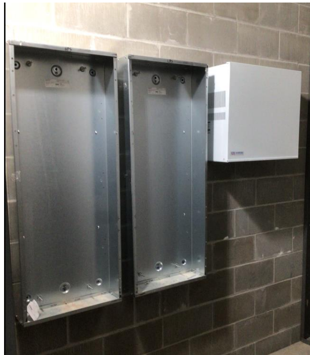
MS South Addition Electrical Panels
