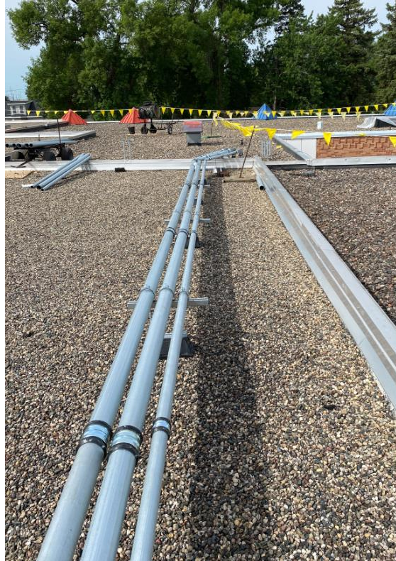
Rooftop Electrical Runs
