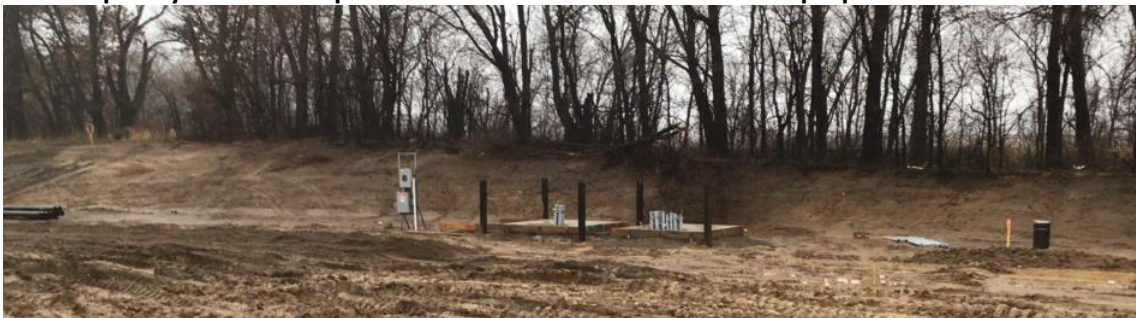
Temporary Power set up and Connexus was out to the site to prepare for Transformer
