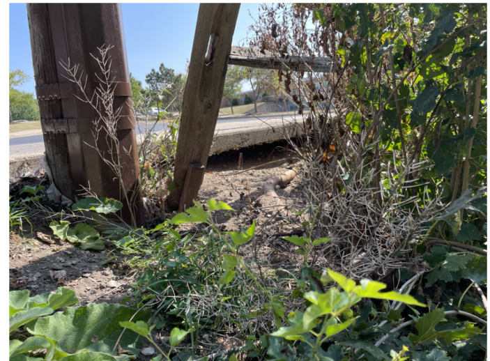
② SIDEWALK UNDERMINING, FENCE FAILING
