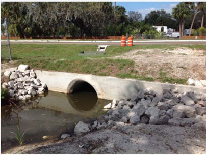
Drainage structure south side of Kracker Avenue
