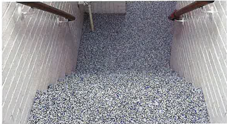
Veregy upgraded deteriorating conditions with new epoxy resinous flooring, new paint, new showers, and new lockers in two locker rooms at Heritage High School.
