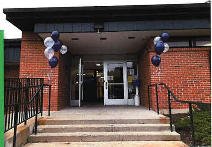
The front entrance at many of the schools were modified with updated ADA compliant ramps and fencing. The fascia at Oak Crest Elementary was also replaced due to deterioration, giving a facelift to the exterior.
