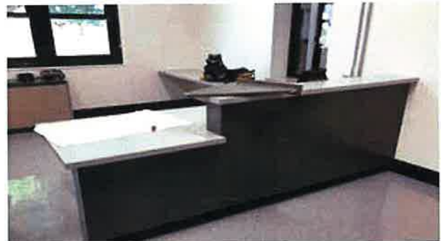
The main office was renovated as Veregy installed new floors, greeting desk, sliding window, ceiling tiles, LED lighting, A/C, and paint.
