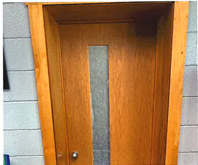
Interior doors were replaced with solid-core prefinished wood doors and the secure door functions were reinstalled.
