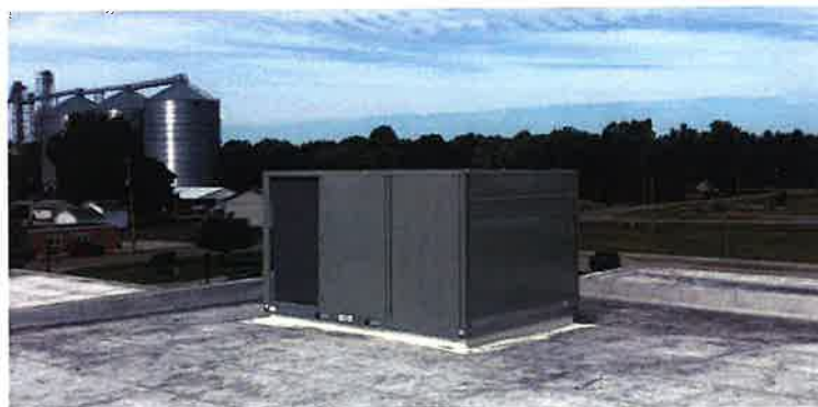
Veregy installed two new energy efficient HVAC roof top unit systems at Heritage Elementary and Junior High.
