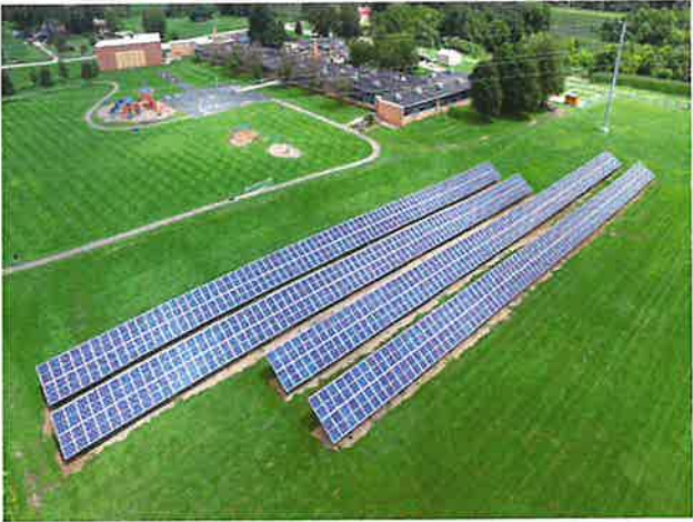
Solar PV Panels at Harmony Emge SD 175
