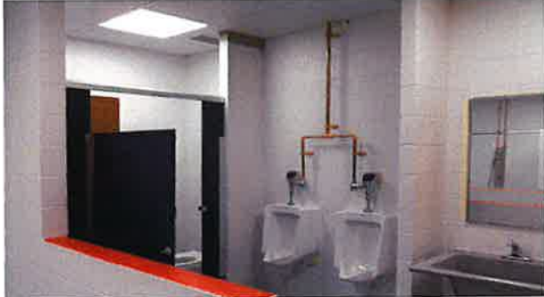
The bathroom was renovated as Veregy installed new floors, partitions, sinks, LED lighting, and paint.
