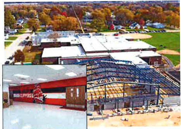
Veregy managed the construction of a new gymnasium with an energy efficient HVAC system and ADA compliant facilities.
