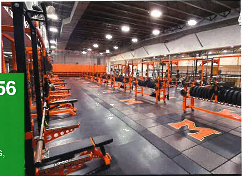
The weight room at McHenry CHSD 156 High School was updated with energy efficient LED lighting.
