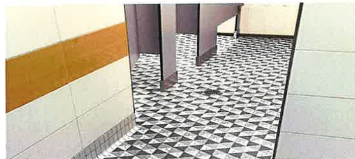
Bathrooms were renovated with ADA compliant stalls and sinks plus new plumbing, LED lighting, hand dryers, stalls, flooring, ceilings, and paint.
