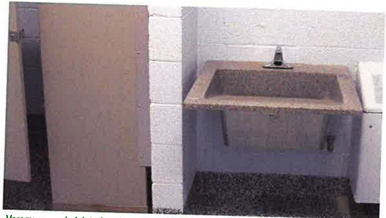
Veregy upgraded deteriorating conditions with new Bradley sinks, epoxy resinous flooring, new paint, new LED lighting, and new acoustic ceiling tiles in four bathrooms at Heritage Elementary and Junior High School.
