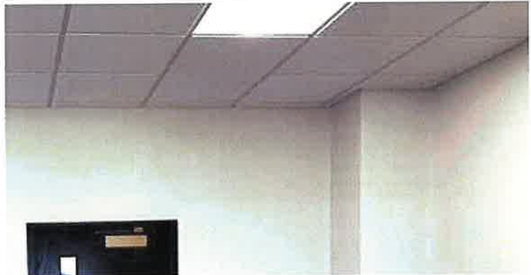
Veregy installed energy efficient LED lighting and new acoustic ceiling tiles in Phase 3.
