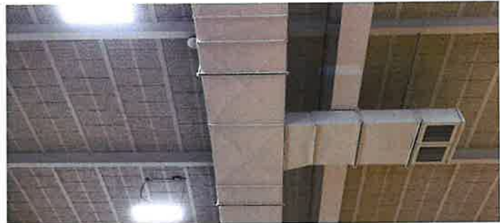
New HVAC systems were installed at each school allowing energy efficient school-wide air conditioning to be available.
