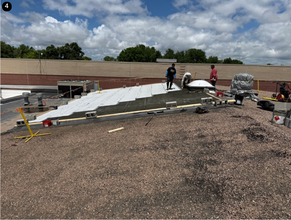
Northeast section has been removed and replaced with base and cap sheet.
