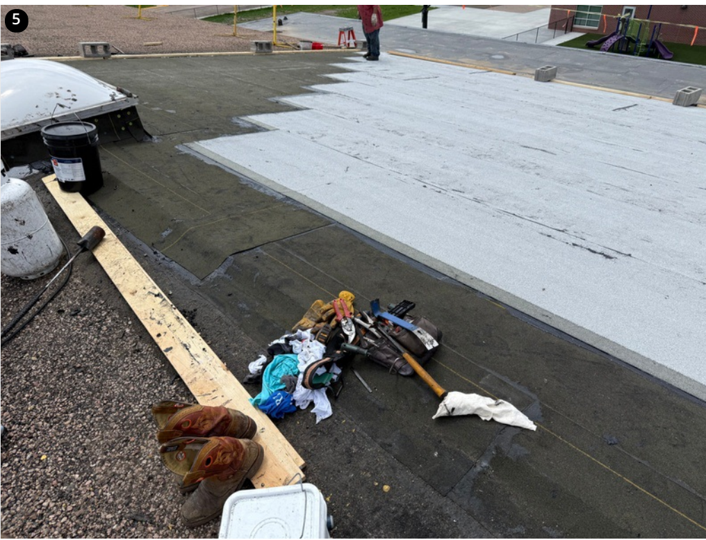
Example of both base and cap sheet being installed. Proper adhesion rates and bleed-out along all lap seams.
