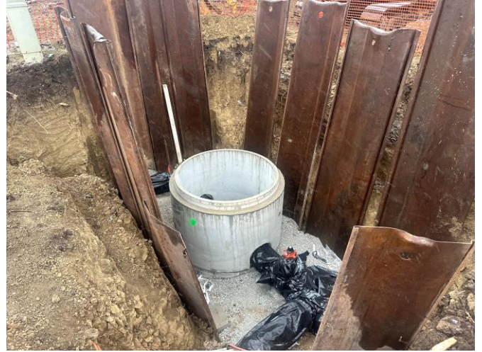
3/11: Check valve assembly and manhole base installed at the water tower site.
