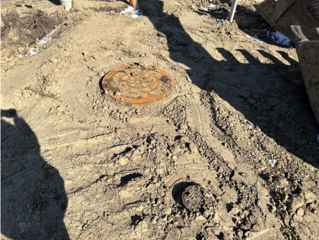
3/16: Manhole cover and valve boxes at check valve assembly near Water Tower.
