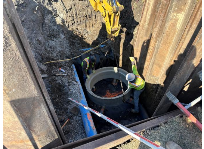
3/16: Set manhole base for check valve assembly on South 68th Street north of the roundabout.
