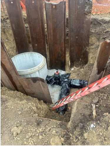
3/11: Check valve assembly and manhole base installed at the water tower site.
