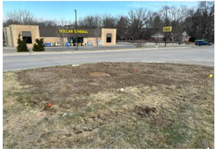
3/20: Manhole cover and valve boxes at check valve assembly on South 68th Street north of the roundabout.
