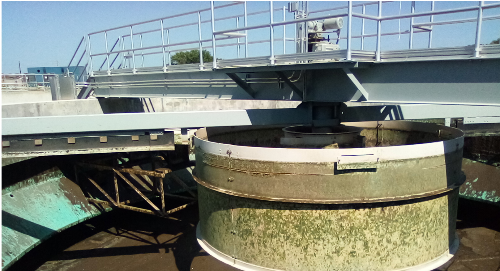
Figure 2: Damage to Paint on Influent Well.
