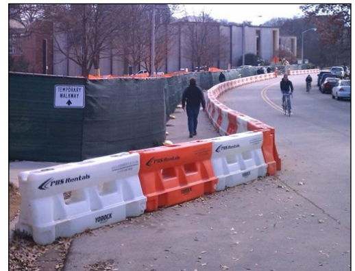
Example of a Temporary Walkway (Source: Yodock.com)
