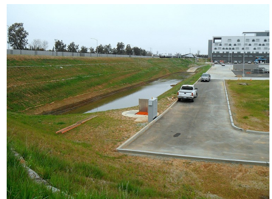
Example of Detention Area for Stormwater
