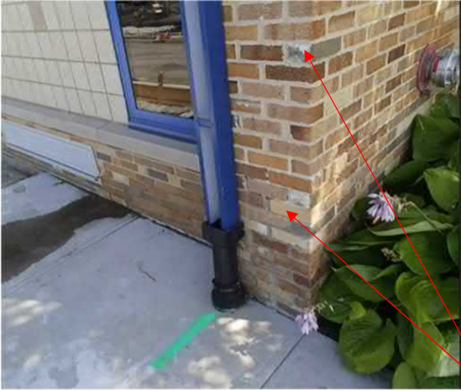
Figure 34: Several bottom courses of brick in need of tuckpointing
