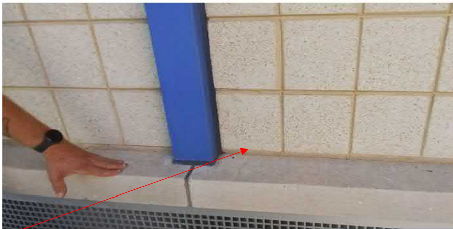
Figure 31: The cast stone sills appear to be 'drooping' at the center of the larger unit ventilator grilles, which is cracking the mortar between the wall and Smooth face CMU window infill. The 1955 and 1993 details show steel lintels for the smaller grilles, but none were found for the larger grilles. Further investigation is required.
