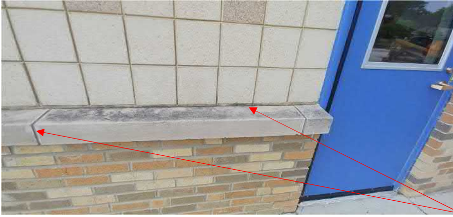
Figure 3: Existing Cast Stone Sills, in need of cleaning, sealing, grinding out of joints and re-sealed with elastomeric sealant, per current construction methods.
