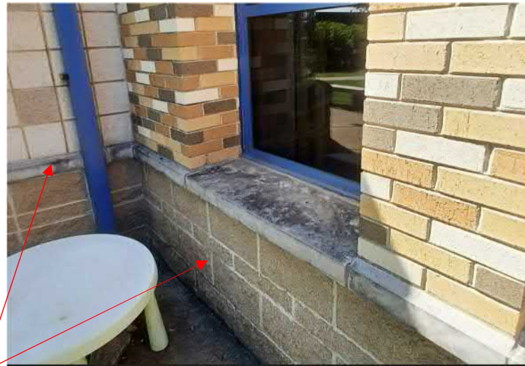
Figure 19: Stained stone sills. Stained stone sills in need of power-washing and grinding out of joints and re-sealing. Areas of split face CMU in need of repair and tuckpointing..
