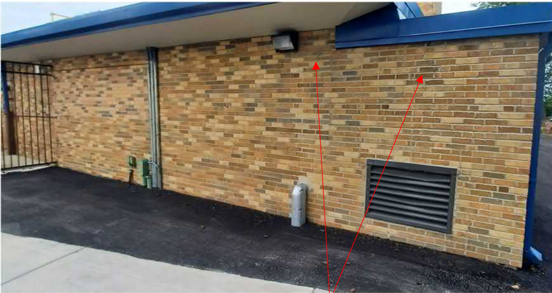
Figure 6: General areas in need of tuckpointing and cleaning.
