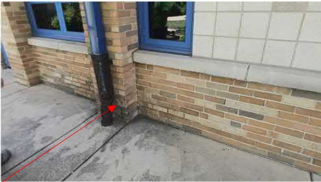
Figure 25: Brick pier in need of cleaning and tuckpointing.
