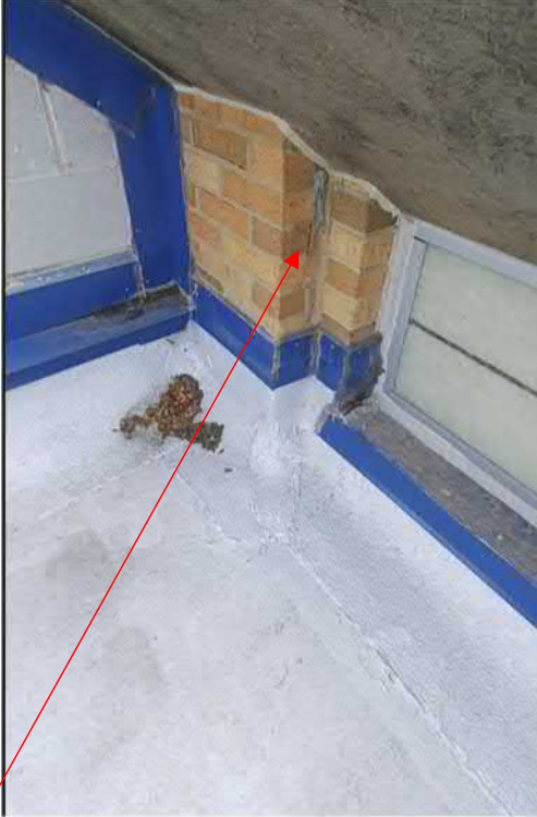
Figure 48: Cracked mortar requiring repair and or replacement.
