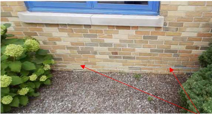
Figure 35: Bottom 2 or 3 courses of brick in need of tuckpointing.
