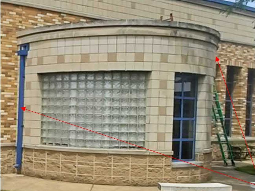
Figure 22: 'Rotunda' area Stone sills in need of grinding out and sealing of joints. Cracked mortar joints in split face and smooth face CMU in need of tuckpointing.
