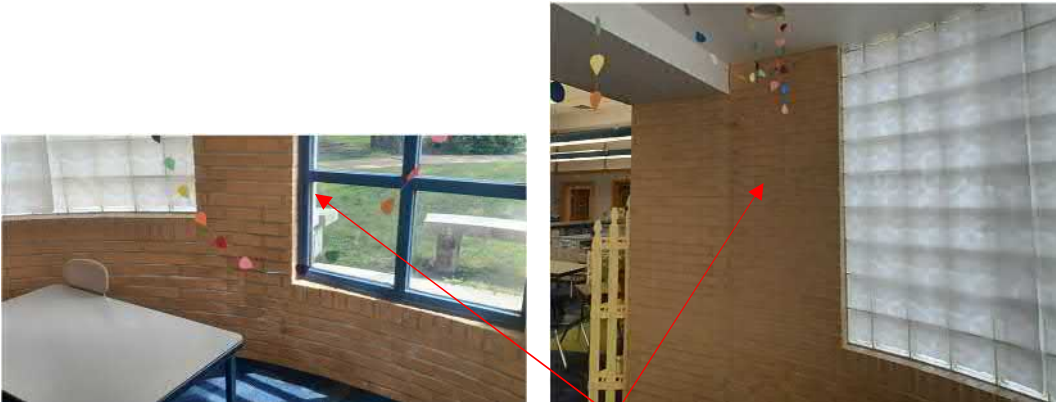
Figure 21: Evidence of water infiltration / efflorescence.
