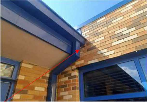
Figure 24: Broken brick in need of repair.
