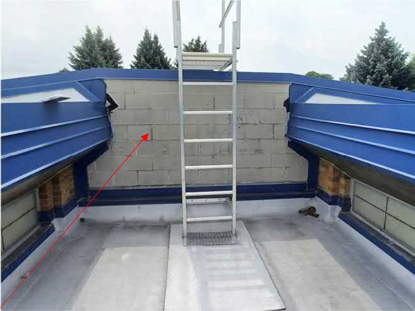
Figure 44: Painted CMU in need of tuckpointing and re-painting.
