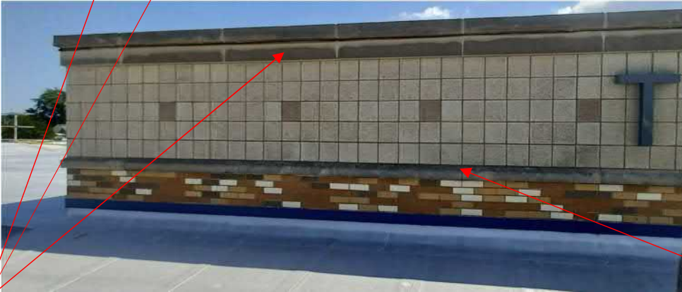
Figure 43: Stone sills and smooth face CMU in need of power washing. Stone sills joints in need of joints being ground out and re-sealed with elastomeric sealant.
