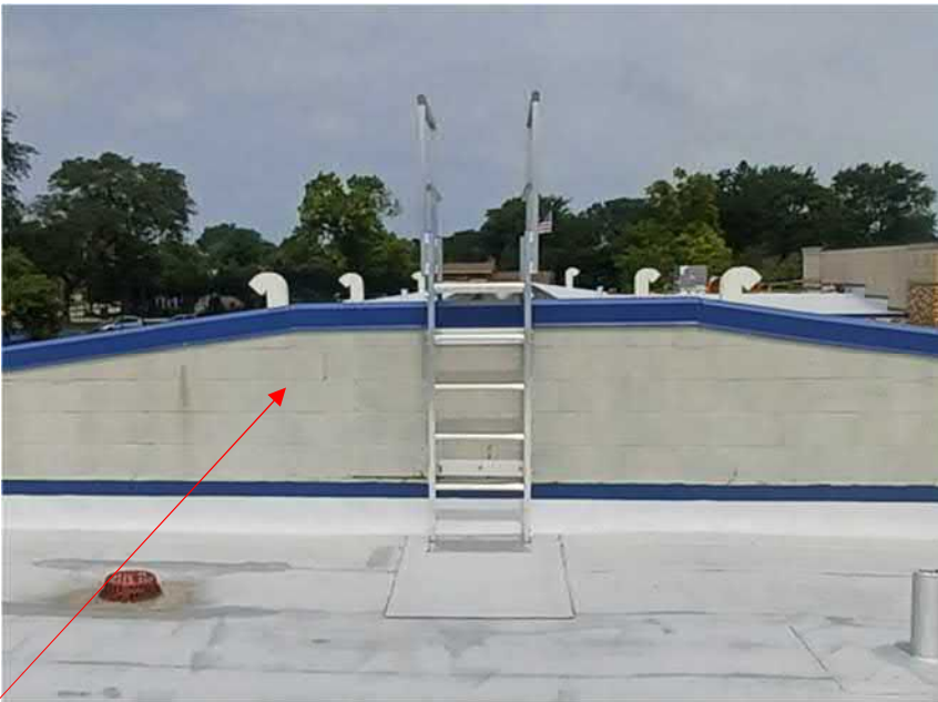
Figure 45: other various areas of painted CUM walls, in fair condition. Future tuckpointing and painting (or covering with metal panel.) should be considered.
