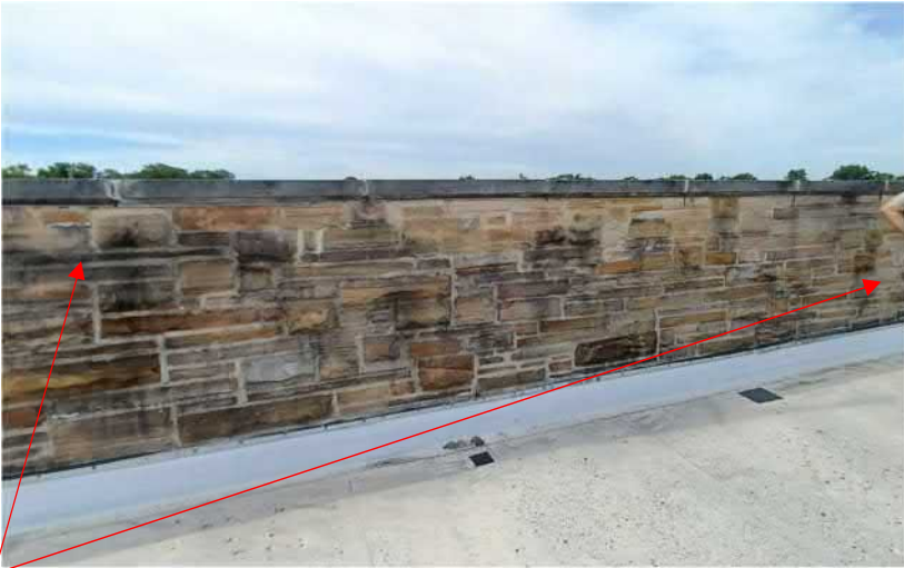
Figure 14: Limestone parapet and wall in need of power washing and tuckpointing. (Note: Existing stone cap to be capped in metal, in base bid master planning roofing work on roof #3.)
