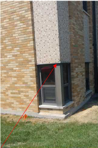
Figure 2: Some tiles coming off at the base that need to be replaced with new. All tile accent fields in need of a 'mortar wash'.
