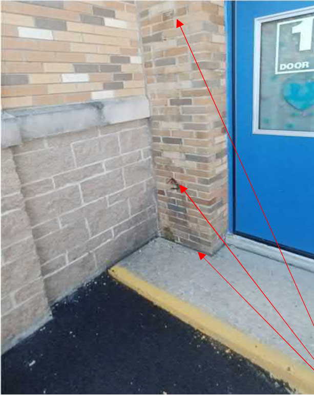
Figure 11: Stoop coming away from bldg. should have compressible filler installed and then sealed. Brackets could be removed, brick pier in need of repair and tuckpointing
