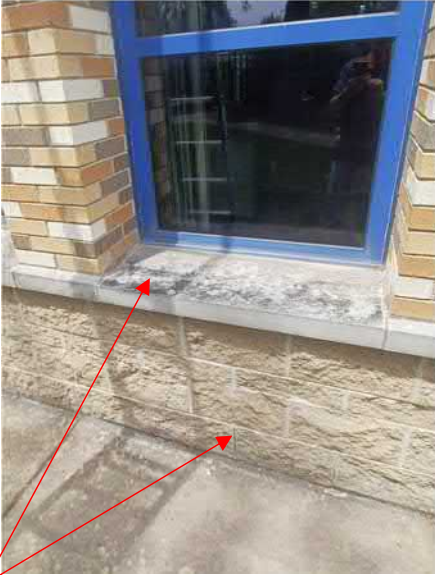
Figure 18: Stained stone sills in need of power-washing and grinding out of joints and re-sealing. Areas of split face CMU in need of repair and tuckpointing.
