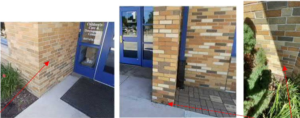
Figure 33: General areas of cracked, broken brick in need of replacing and tuckpointing.
