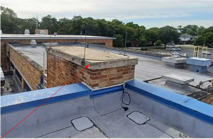
Figure 12: Deteriorating stone chimney cap, (To be replaced in base bid master planning work.)
