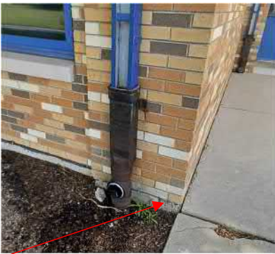
Figure 16: Foundation wall in need of repair.
