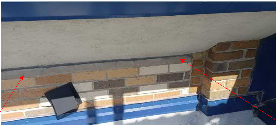
Figure 47: Cracked mortar requiring repair and or replacement. Tuckpoint all broken and open joints.
