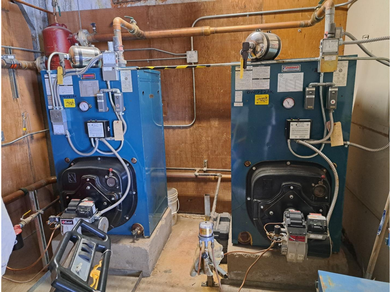
Figure 2 All boilers are set up the same throughout the district
