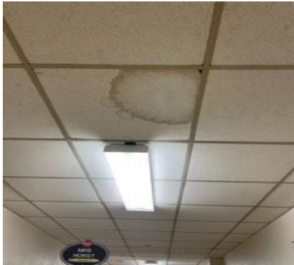
Stained and dated ceilings
