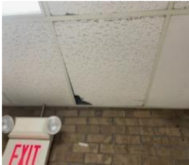
Stained and dated ceilings
