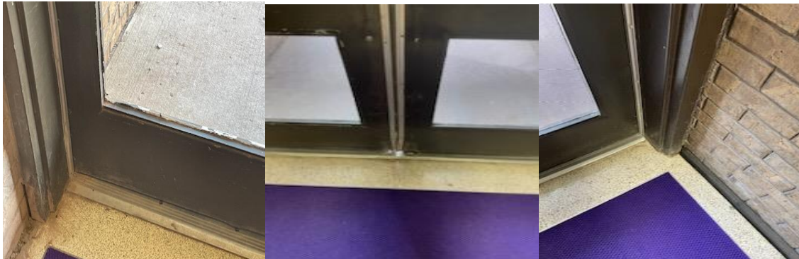
Exterior Door Deterioration
