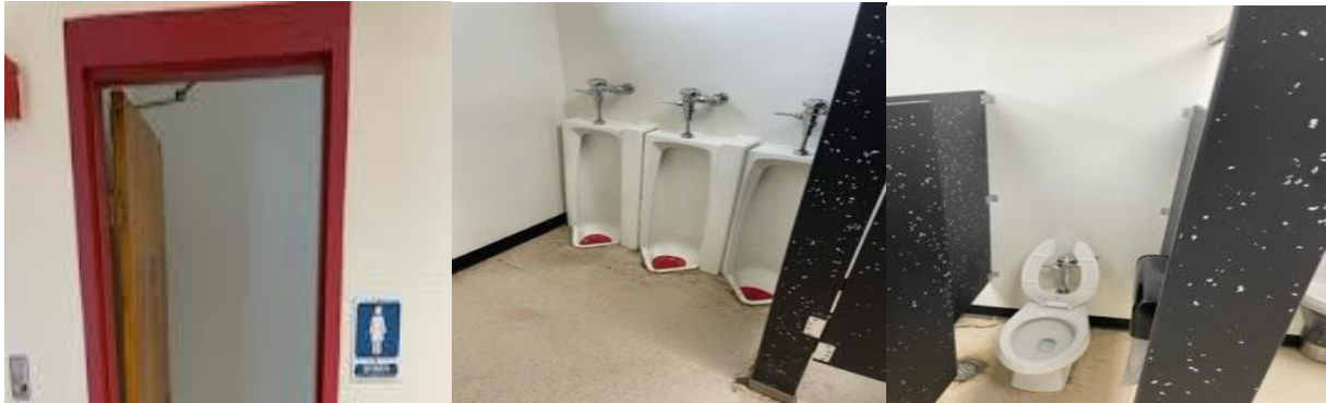
Dated and lack of ADA accessibility (original wing) in restrooms
