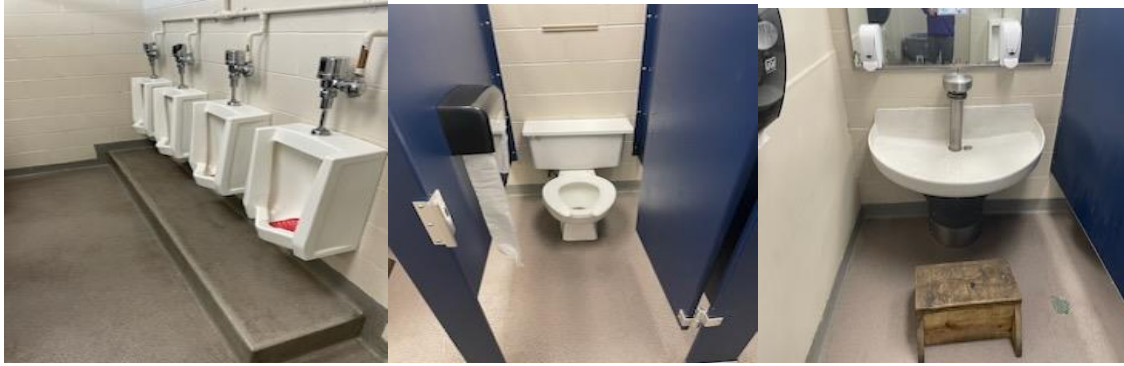
Dated and lack of ADA accessibility in restrooms
