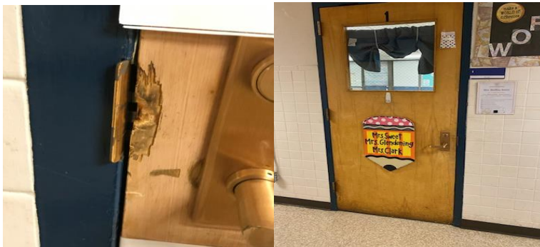
Dated and deteriorating doors
