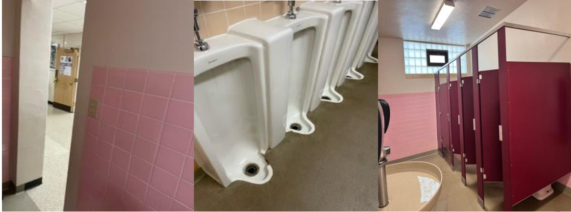
Dated and lack of ADA accessibility in restrooms
