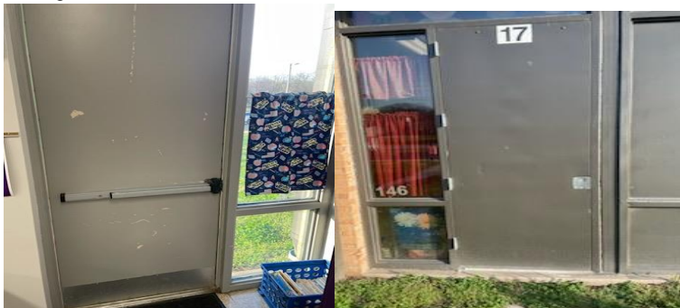
Exterior door frames deteriorated
