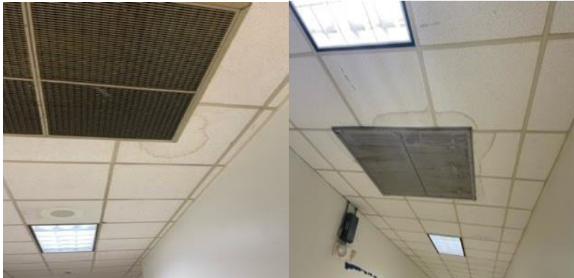
Stained and dated ceilings (original wing)
