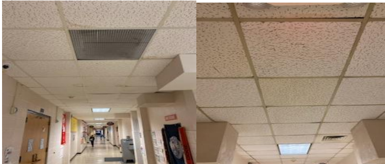
Stained and dated ceilings
