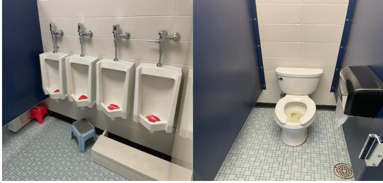
Dated and lack of ADA accessibility in restrooms
