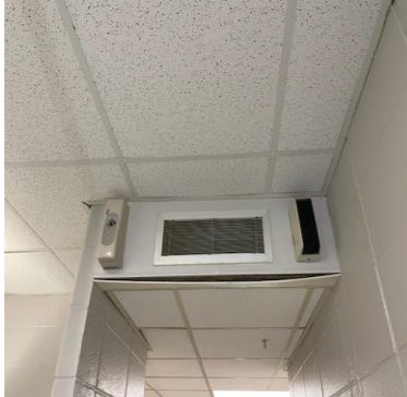
Stained and dated ceilings
