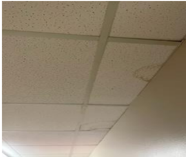
Stained and dated ceilings
