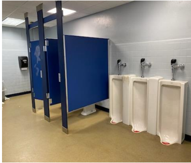
Damaged and lack of ADA accessibility in restrooms
