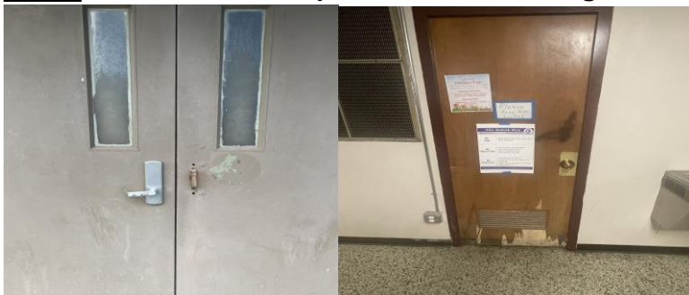
Exterior and interior doors and hardware are deteriorating
