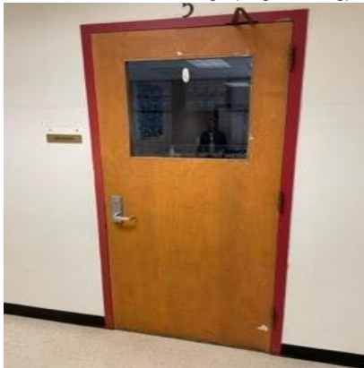
Dated and deteriorating doors (Original Wing)
