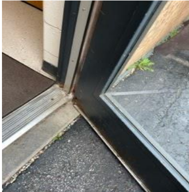
Exterior door frames rusting and deteriorated
