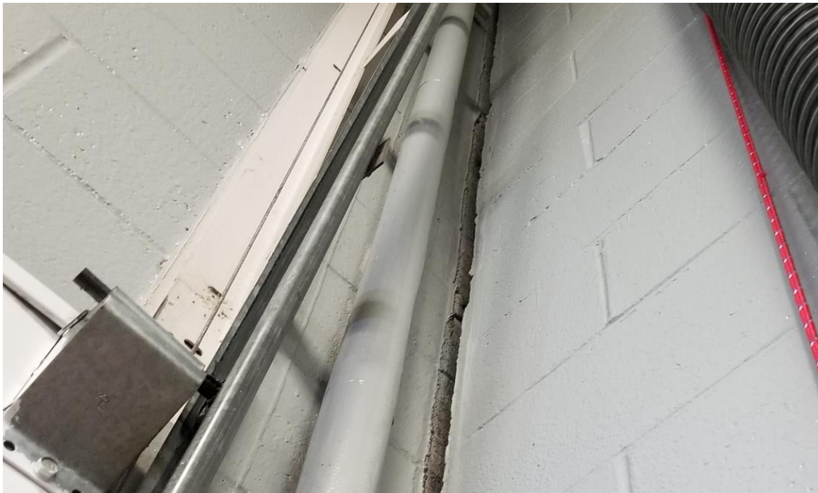
Separation at CMU Wall Intersection
