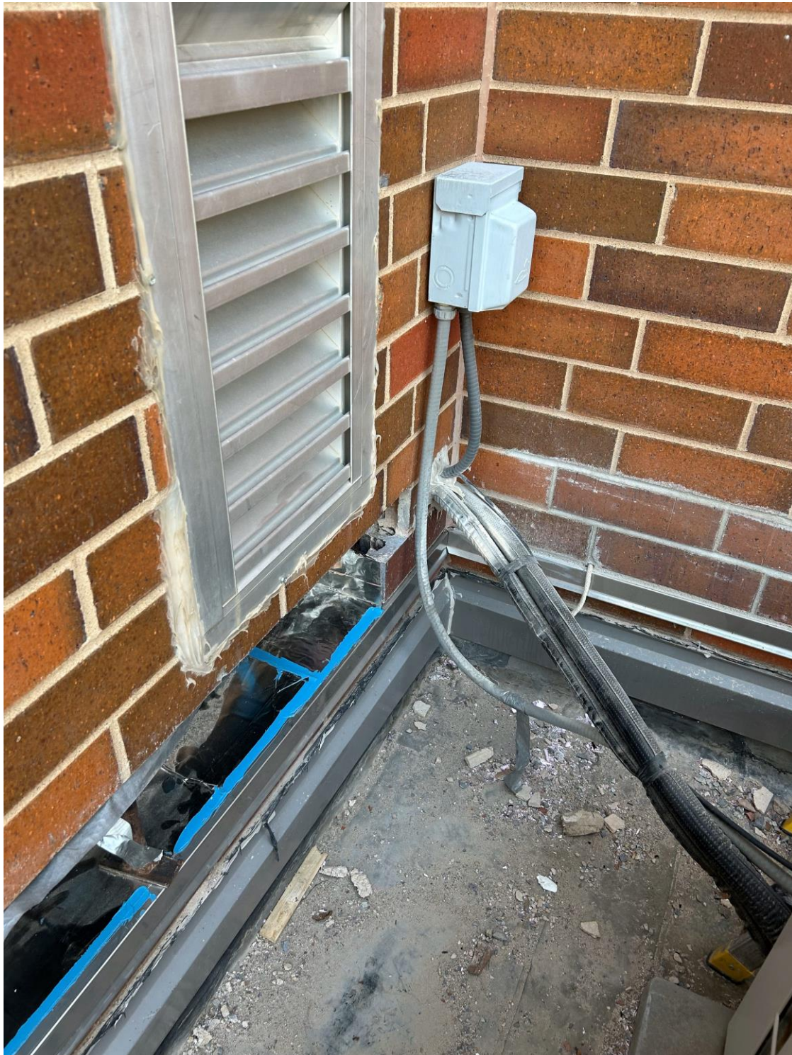
Flash by end dams at the brick are under the condensate line due to mechanical line (Green Area) 49
