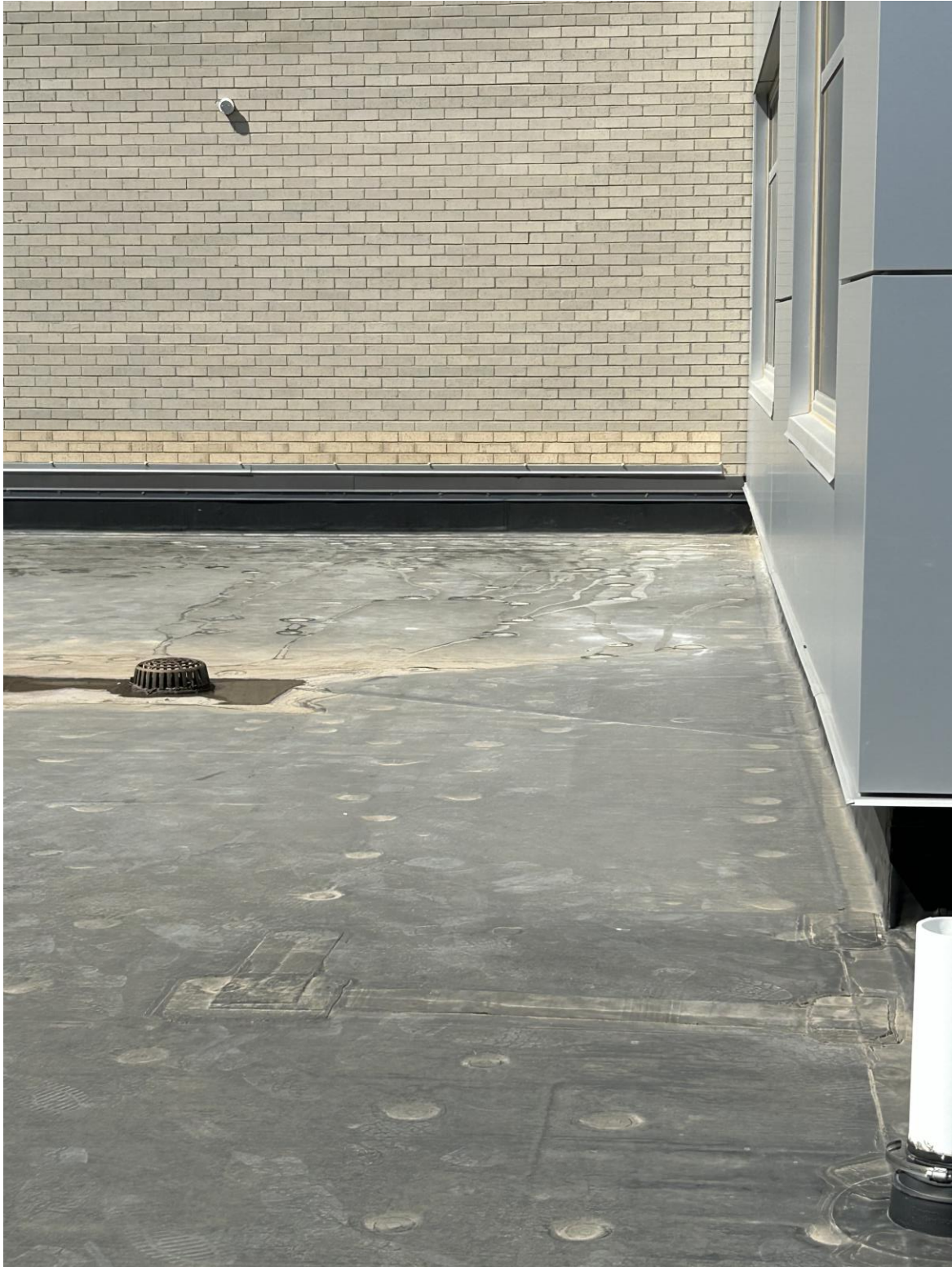
Completed through wall flashing. Bottom 3 courses of brick have been tuckpointed. New Weeps 43 and Reglet.
