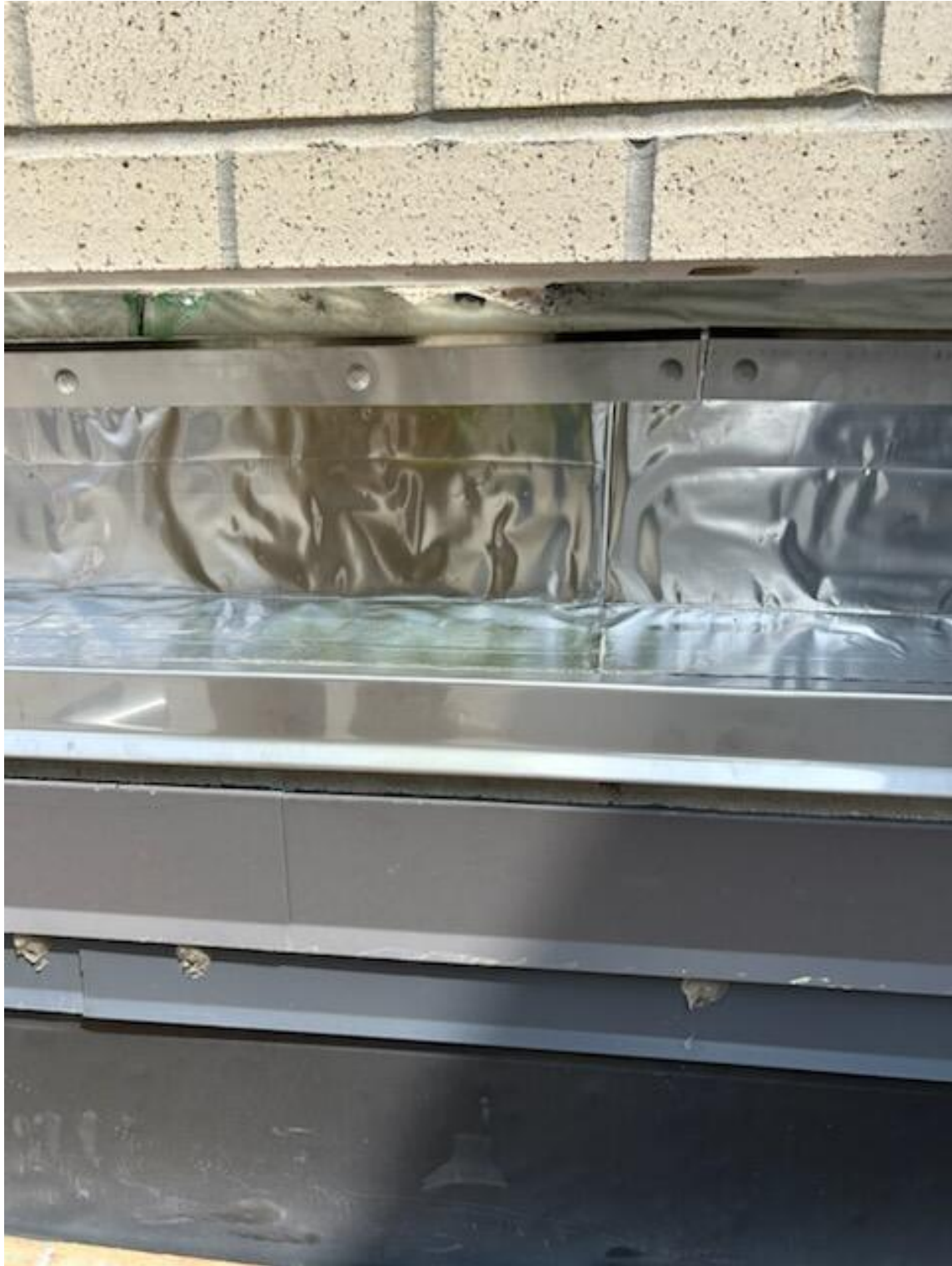
Through Wall Flashing Repair in Progress - 2 Courses of Brick Removed to Install Through Wall Flashing 40 System (Pink Area)
