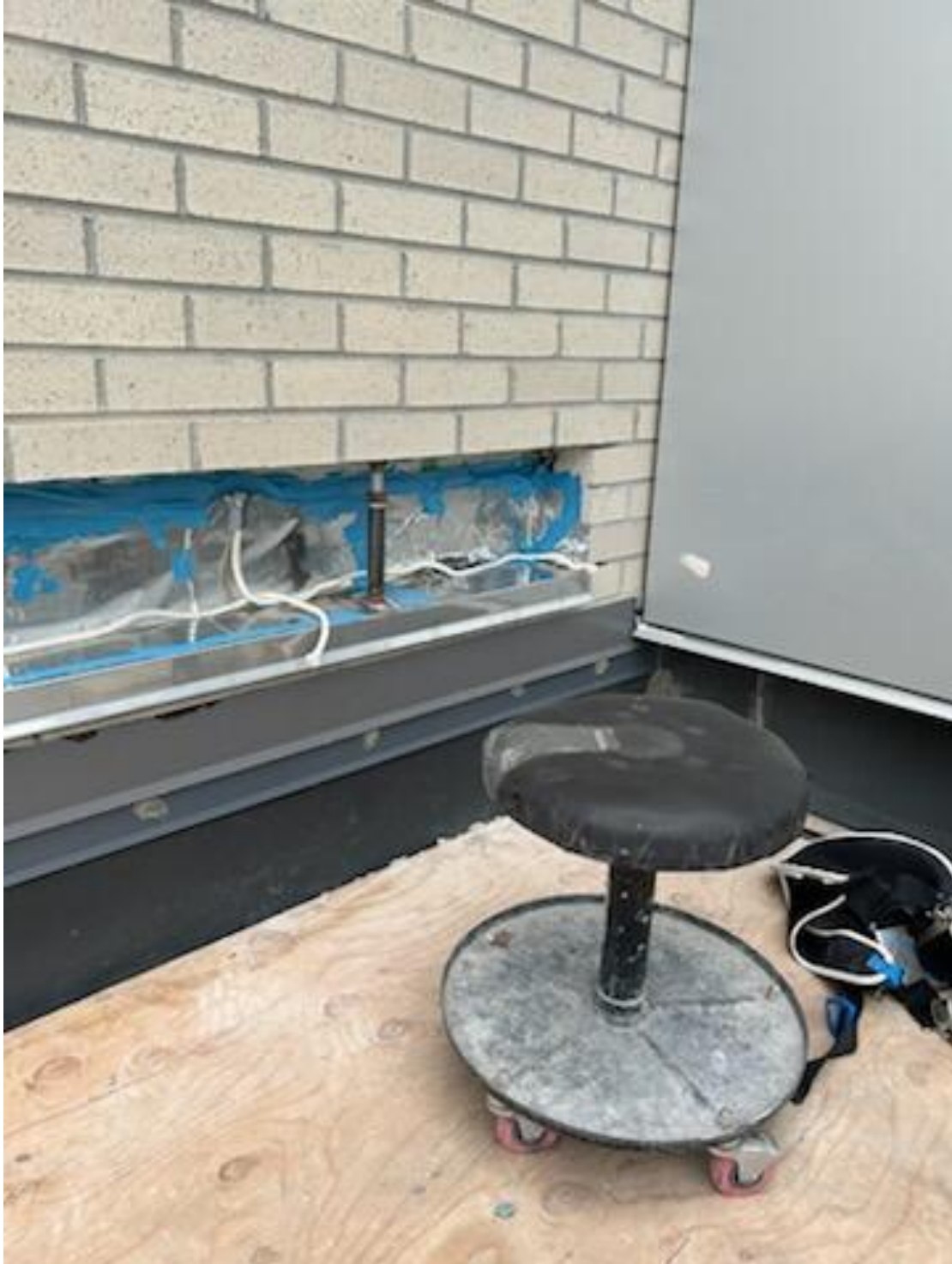
Through Wall Flashing Installation in Progress - New Weeps for Water to Exit the System
