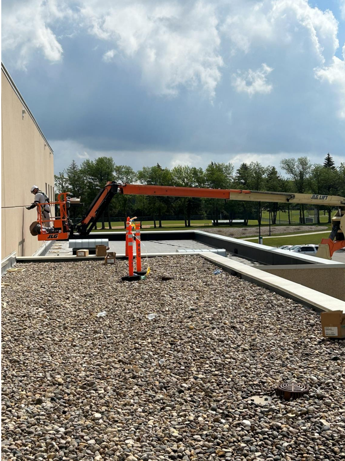
Precast Sealant Replacement in Progress (Orange) Loose residual sealant removed, Replaced with New Urethane Sealant
