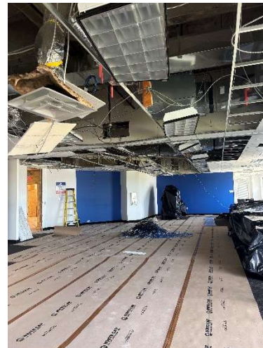
4th Floor – New IT Area Demo
