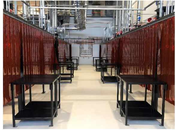
Welding Booths at Trade Bar B
