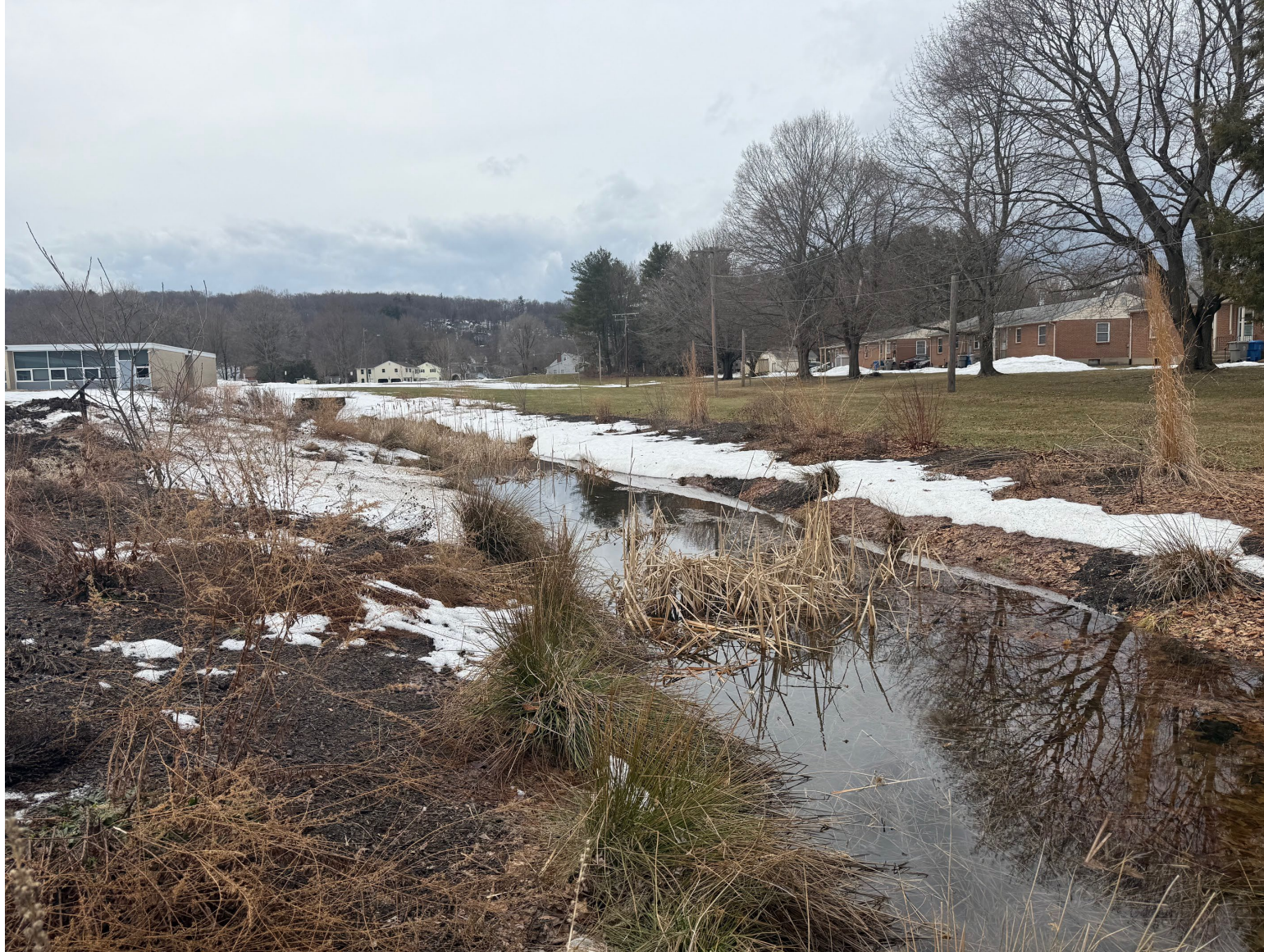
Current view of swale (wetland) north of eastern parking area after bio-swale construction.
