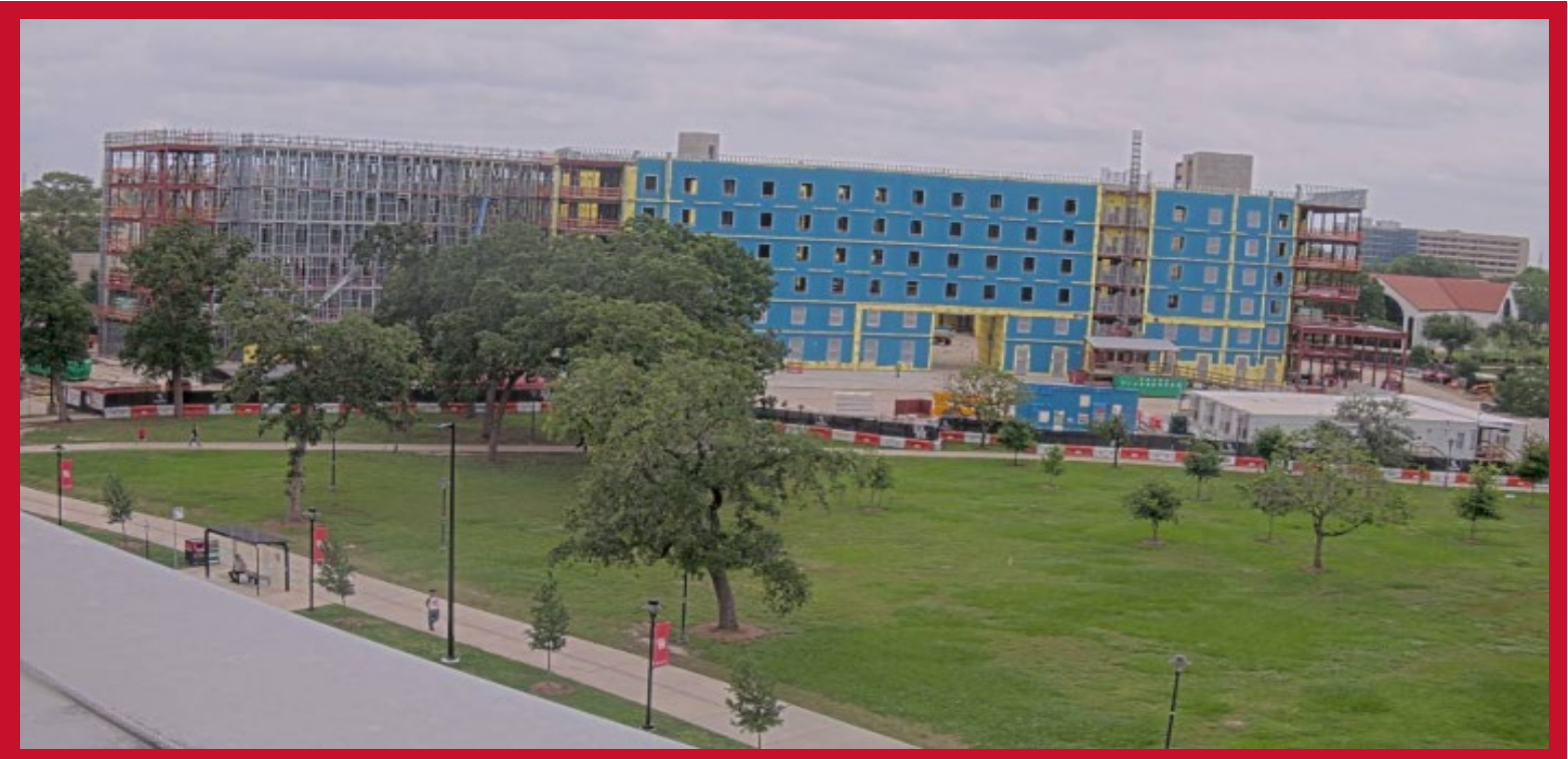
Freshman Student Housing Project - Photo courtesy of University of Houston Information Technology Service Webcams.
