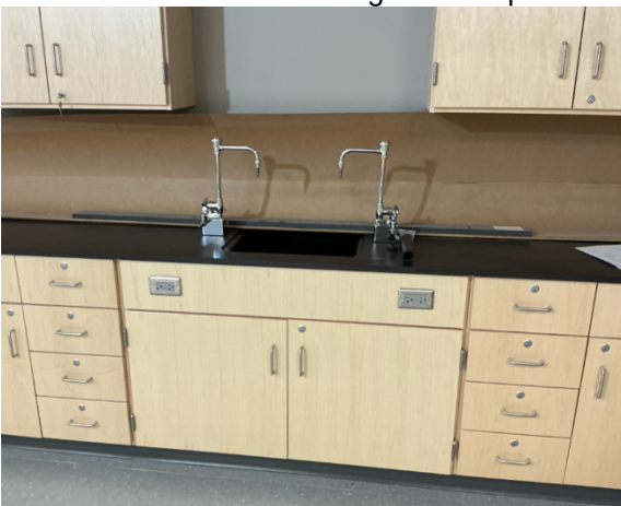
Casework and Plumbing in the Science Room
