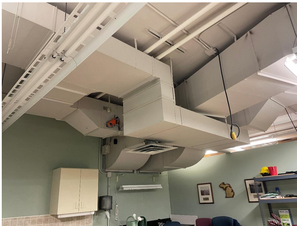
Figure 3: Bypass damper (orange actuator), return branch, and supply/return mains.
