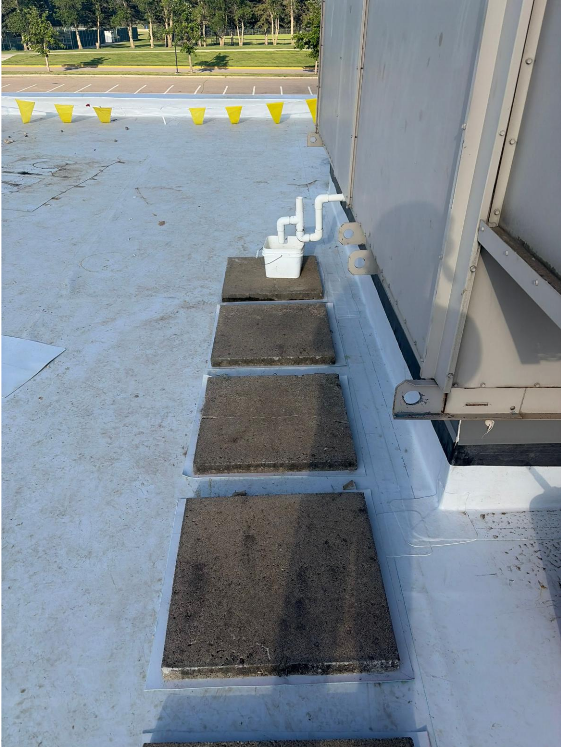
Concrete pads placed around perimeter of unit to capture condensate on roof area #6
